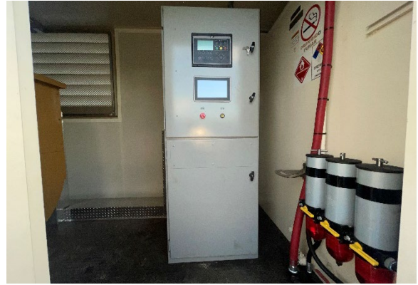
Refurbished CAT EMPC 4.4 Cabinet w/ Paralleling Capability 1250 Gallon Double Wall Fuel Tank
