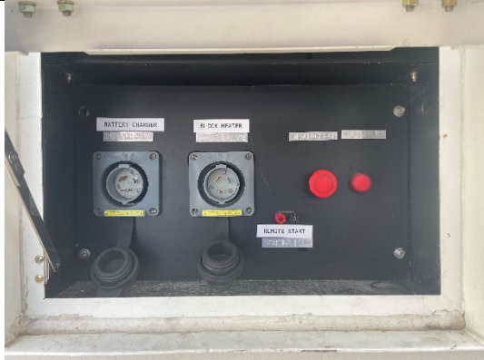
Shore Power, E-Stop, Auto-Start, Live Bus Indication
