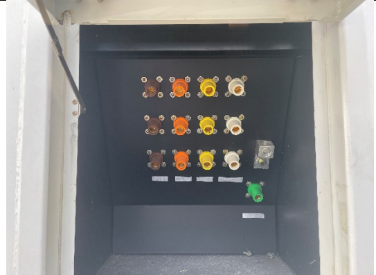
Camlock Distribution Panel
